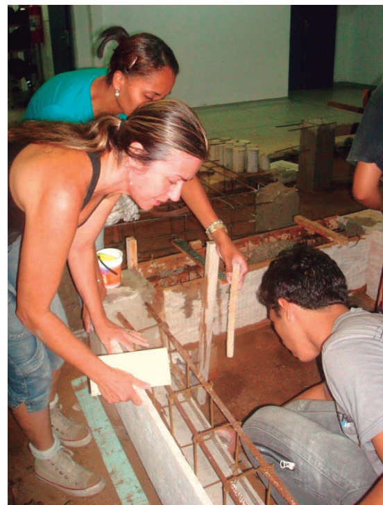
Figure 2 - The students building the structures – Phase 2: putting the steel armour for reinforced concrete
